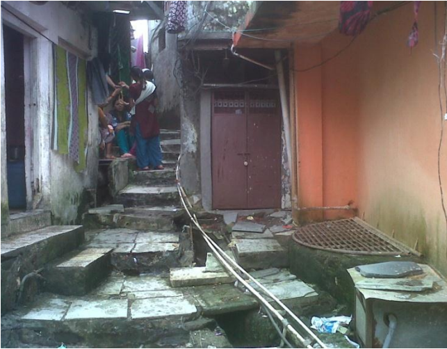
Figure 1 Sewer Lines in Bhandup Slum, Mumbai. Source: Shreyashi Dasgupta, 2014
