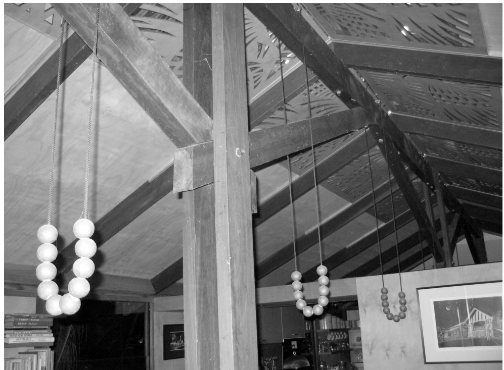
Figure 2. Designing and Matching: Sinkers as Counterweight Cord Pulls for Timber Screens to a Rooflight Vent, Living Room, Taringa House, Brisbane. 23
