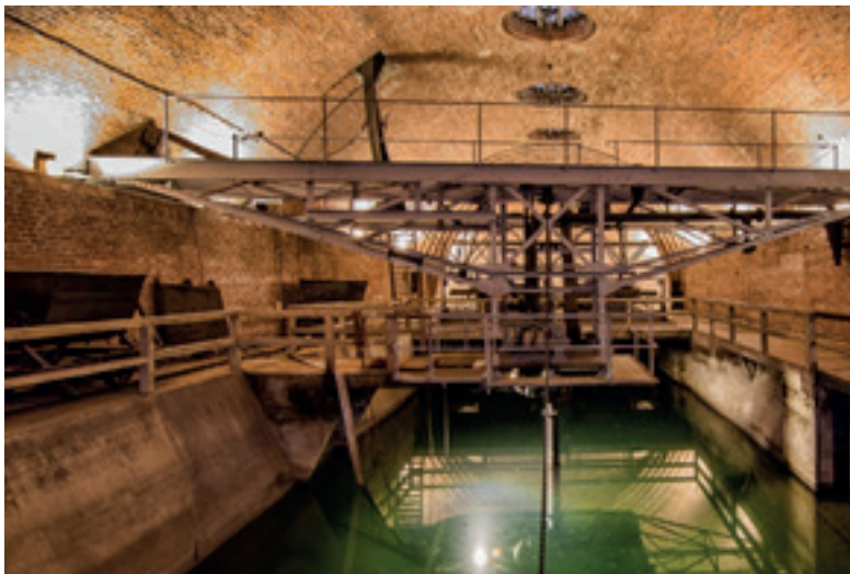
Figure2: Old WWTP, Prague, CZ, The sand trap.
