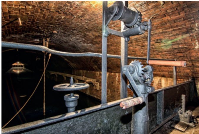
Figure3: Old WWTP, Prague, CZ, The sedimentation tank.
