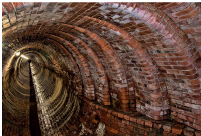
Figure5: Old WWTP, Prague, CZ, The sewage open to public.
