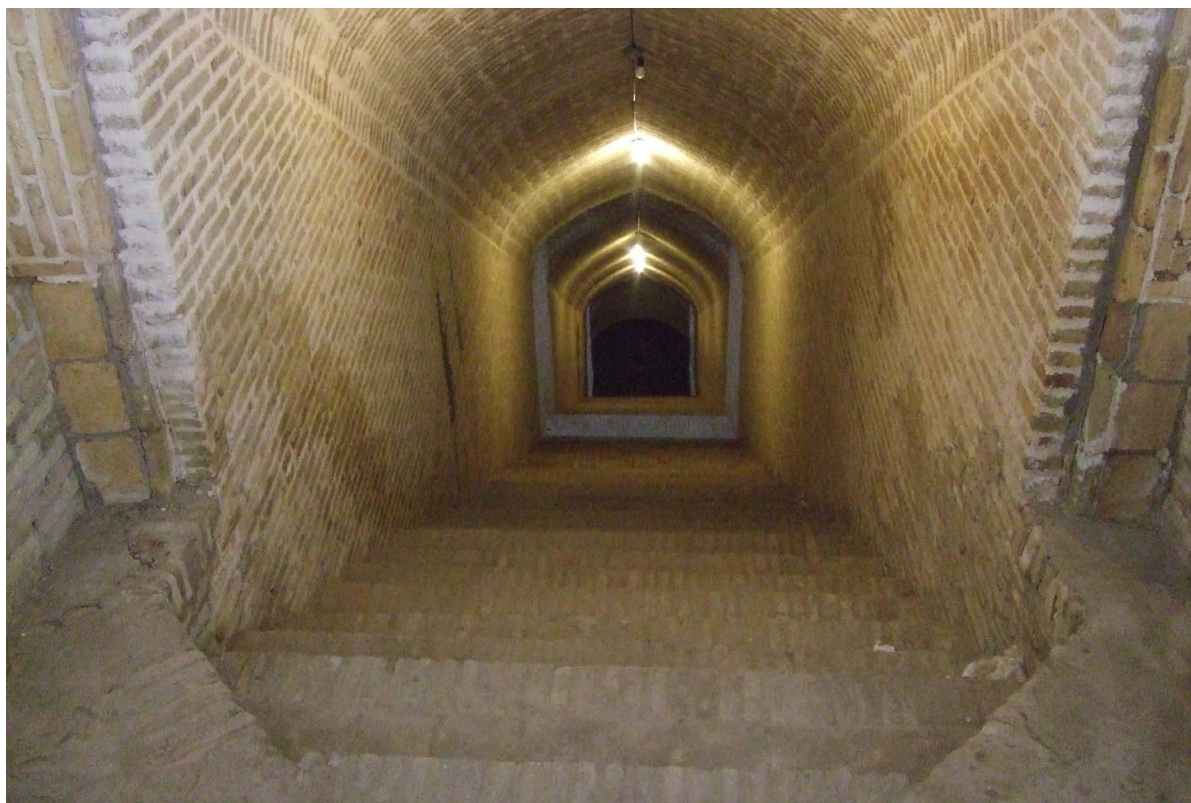
Rehabilitation of a payab, the access gallery to qanāt/kāriz in the urban structure of Yazd (Canavas, 2015).
