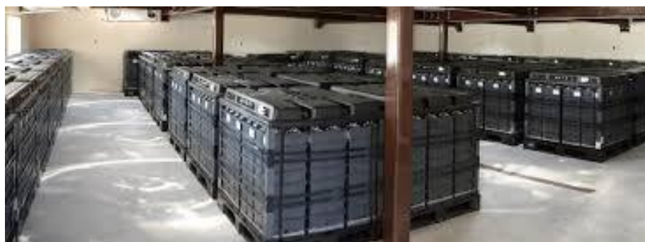
Figure 4: Salt-water battery can power off-grid house.
