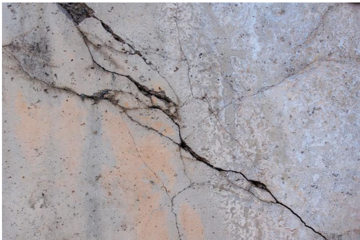
Figure 9: Crack in the wall. It is a figure that cannot be represented by classical geometries. Source: http://www.pixabay.com .
