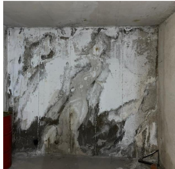
Fig. 6. Visible Moisture on concrete wall without Admixture.
