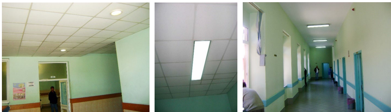
Fig. 7. Different types of luminaires in the corridors (Source: Authors).
