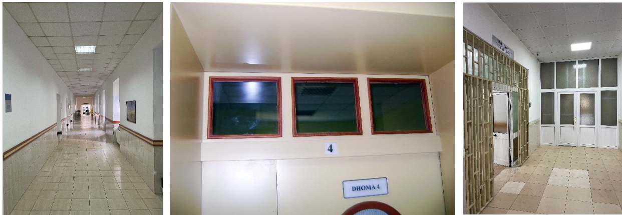
Fig. 6. A. Central mounted luminaries; B.C. Opening in the upper part of the door (Source: Authors)
