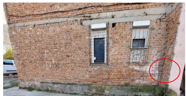
Fig. 13 – Red silicate brick wall façade and mold evidence, Source: Authors.
